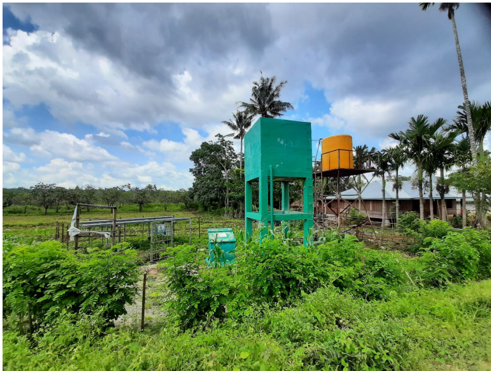
Figure 17: SWP in Bidi Praing and Green Reservoir Added through Village Funds
