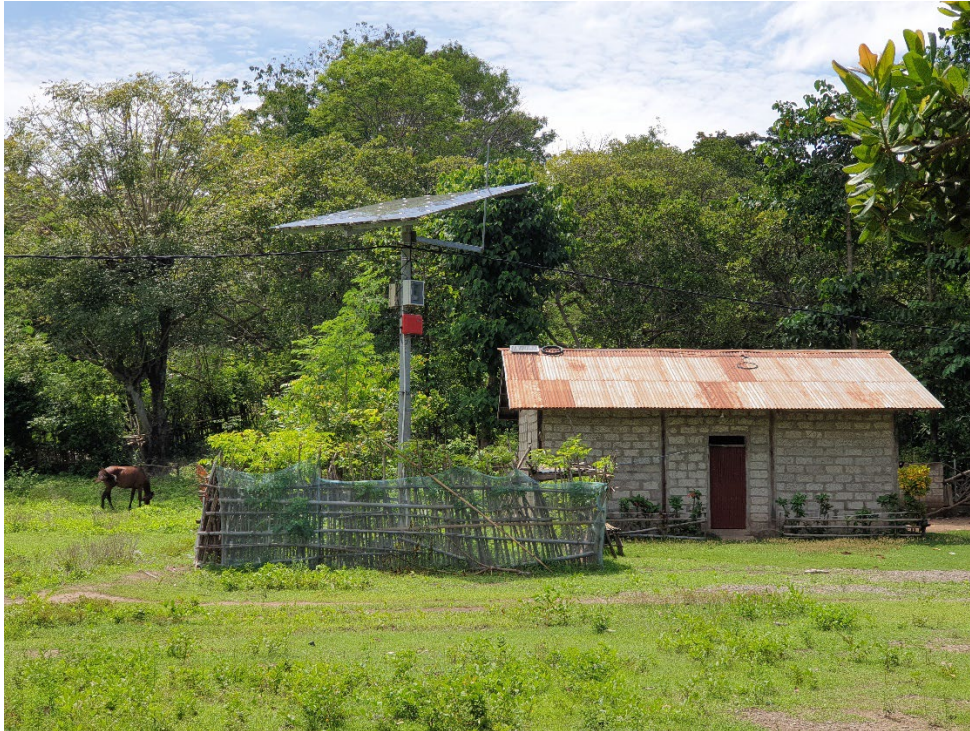
Figure 5: Solar Panel in Praiwitu
