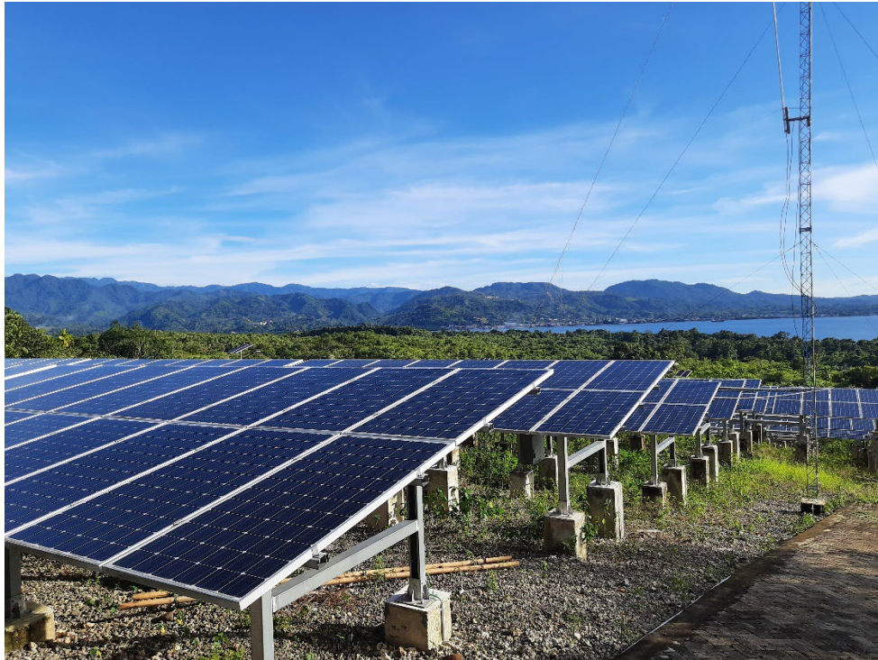
Figure 12: Sky Energy Solar Grid Systems and Beneficiary Households on Karampuang Island
